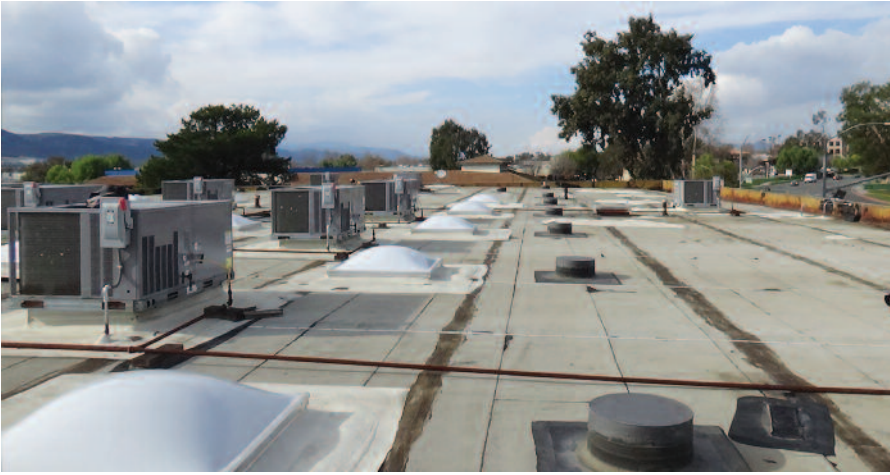
The single-ply membrane on the original BUR roof had been patched many times but was deteriorating and leaking.
