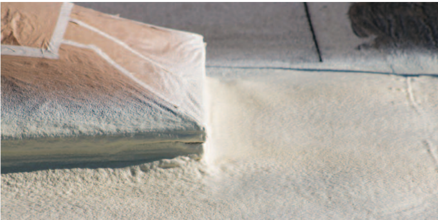
CcSPF's unique ability to contour and seal around skylights and the many other rooftop protrusions made it an ideal solution.
