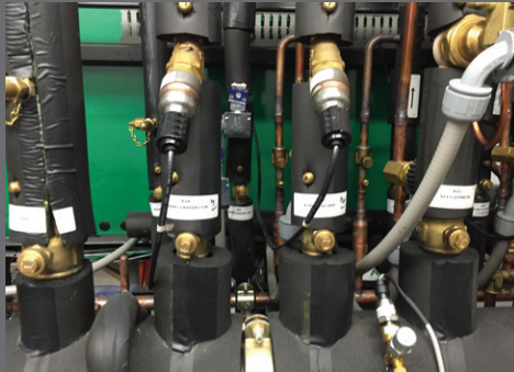
Refrigeration valves on the medium temp refrigeration rack.
