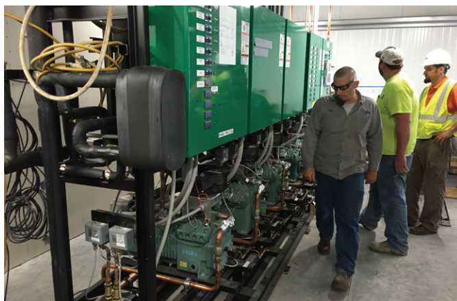
The team from Zero Zone, SCR and Coborn's make final adjustments to the low-temperature rack system.
