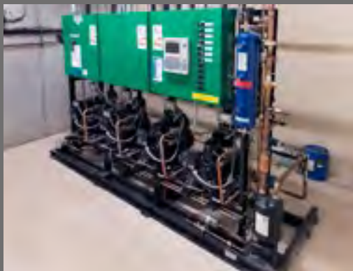
The new refrigeration systems serves the entire store with just 8 compressors on two split-section racks.
